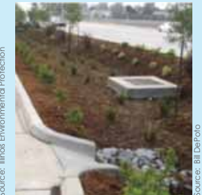
An overflow outlet conveys runoff that exceeds the bioretention area capacity.
